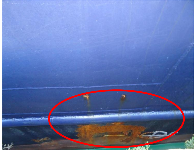
Load lines missing
