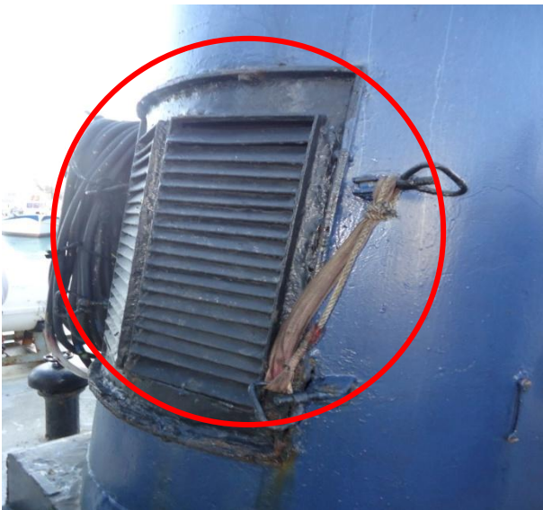
The hatch of the natural ventilator on the funnel (FWD) was missing
