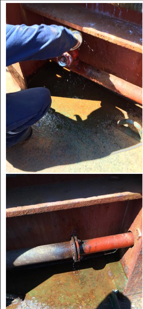
Picture 3: Fire Main Line
