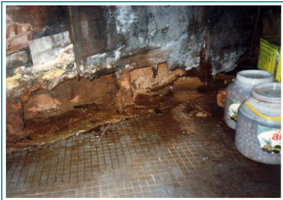
Serious deterioration of insulation in a domestic reefer space constitutes an infringement of ILO requirements concerning food and catering
