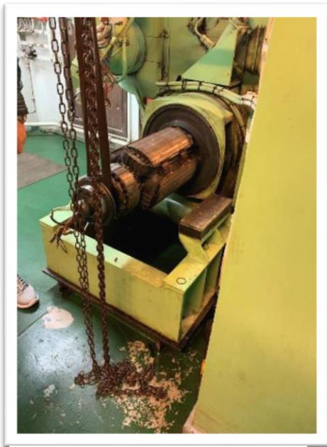
Picture 6: Em.cy Generator
