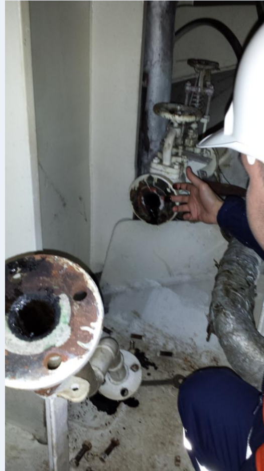
16. Overboard line after three way valve dirty of oil residues (suspected of discharge violation – R.O. responsibility),
