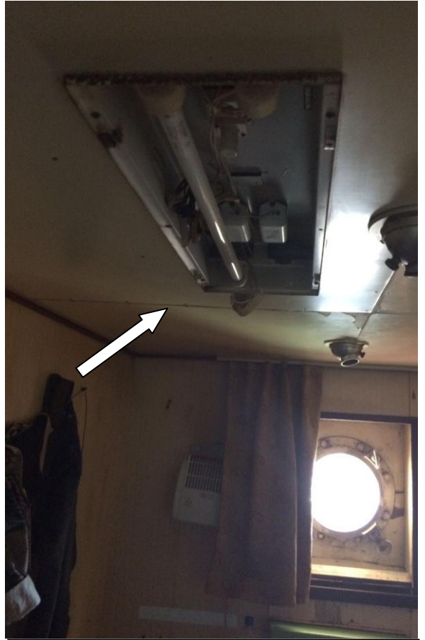
Lamp cover missing in crew cabins
