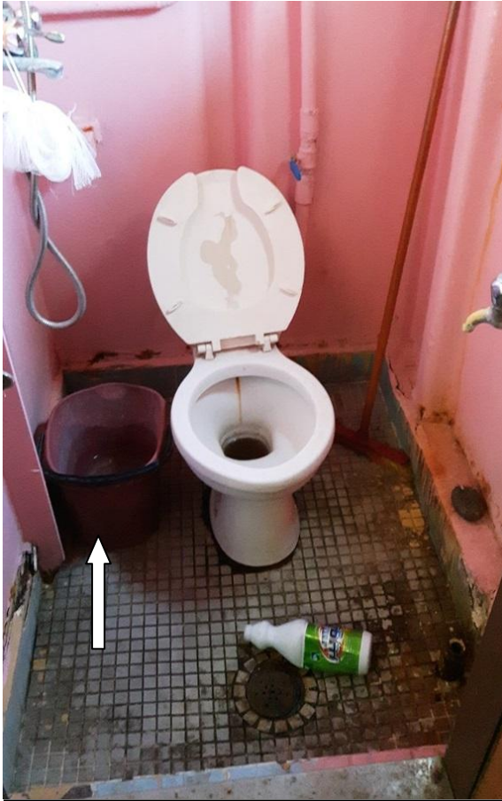
Very poor condition in sick-bay toilet (notice the bin used as flush)
