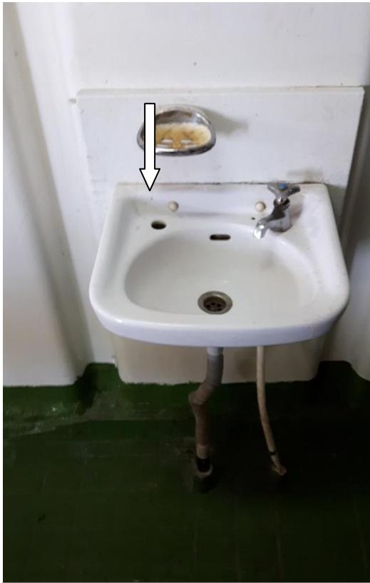
Hot water tap missing
