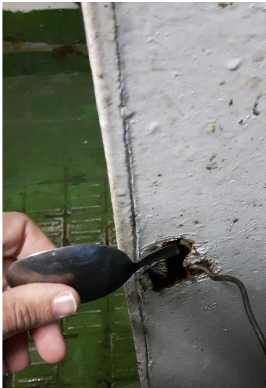
Damaged fire door in galley
