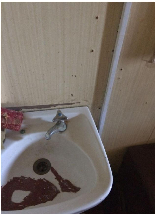
Rusted basin in crew cabin
