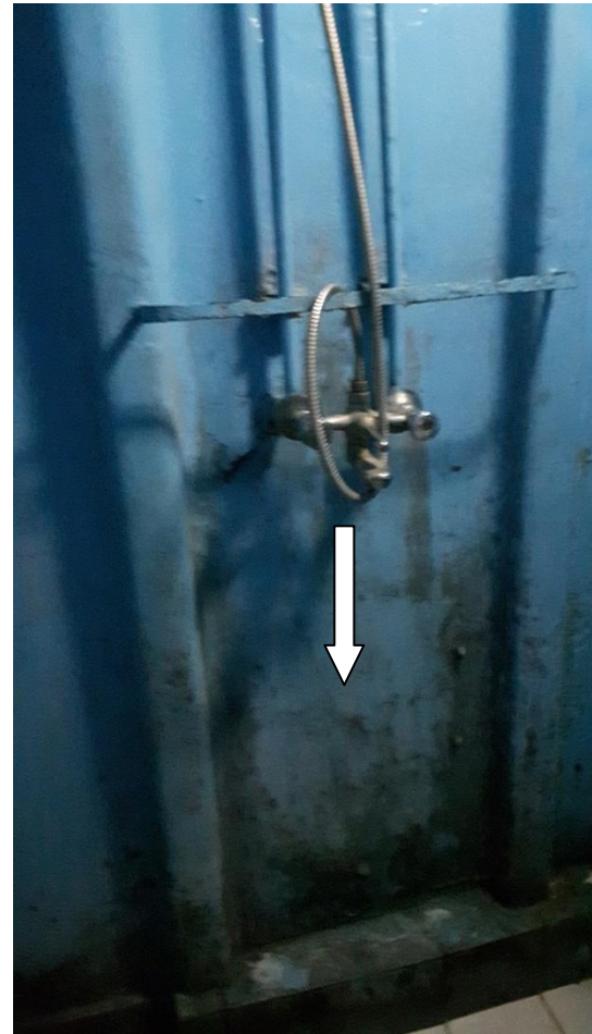
Very poor condition of shower room
